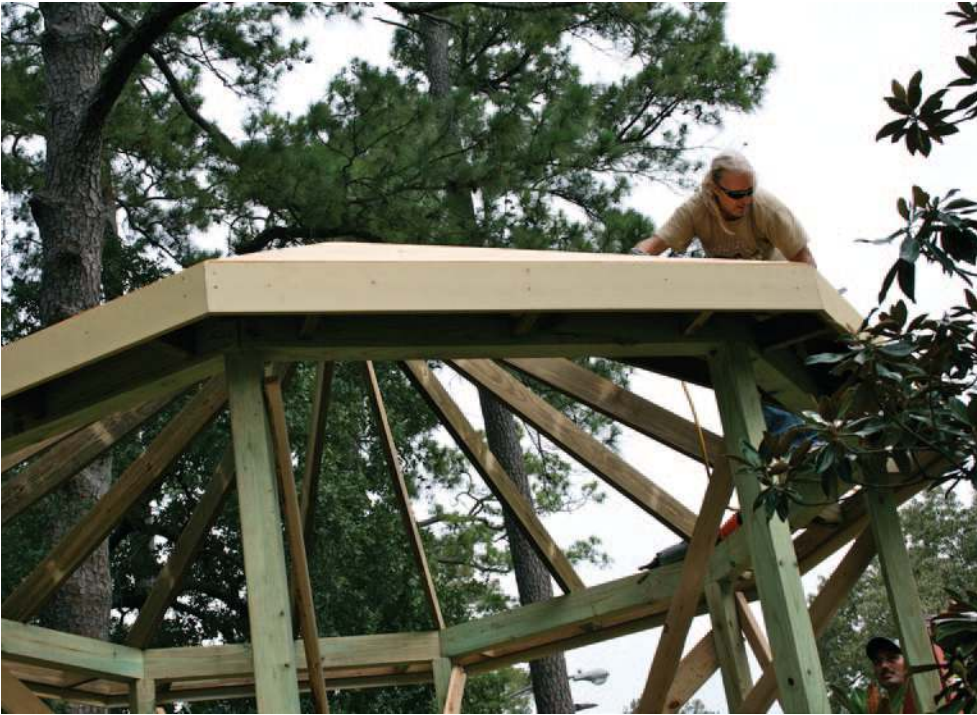
The new Garden Oaks gazebo is rising. The GOCC approved funding the new gazebo at its June meeting. Harry James is donating his craftsmen Rick Wozniak's (shown above) time and providing the materials at cost.
